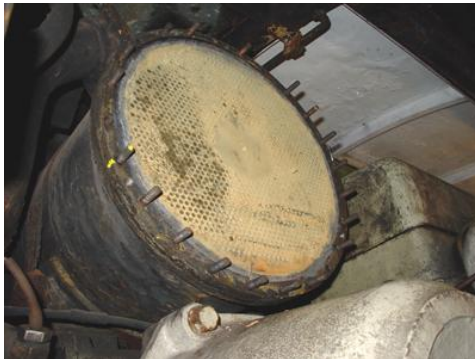
Intercooler with end cover removed for cleaning.
