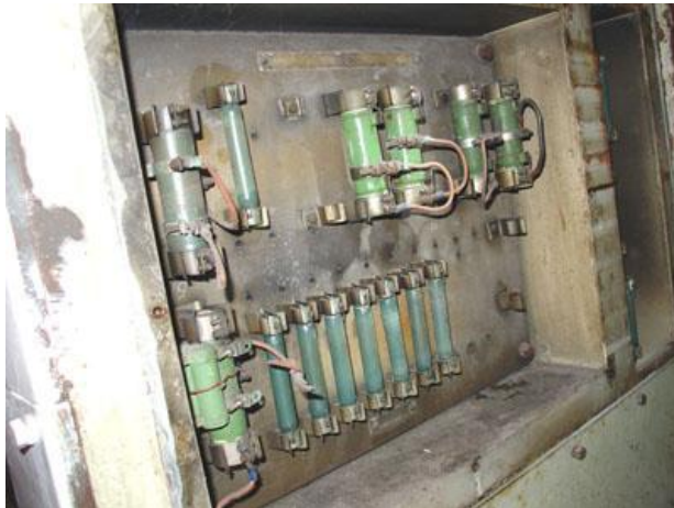
Damaged resistors and clips that will need replacing.
