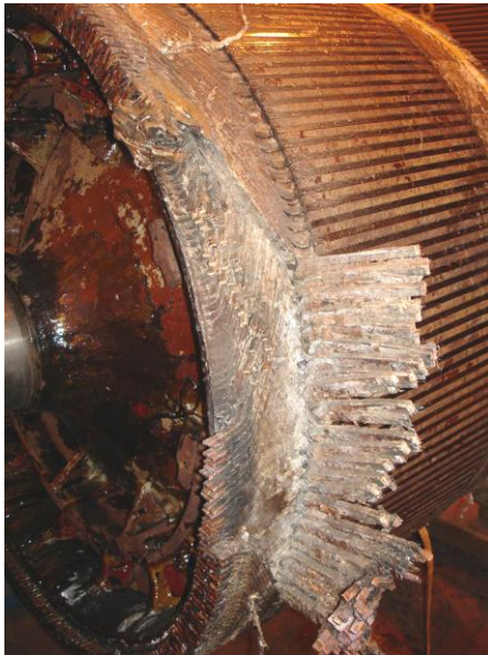
Majority of damaged windings now pulled back and ends cropped. Photo by Mike Jacob.
