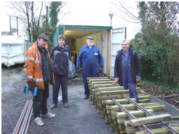
Chris, James, Keith and Martin on track panel production duties 21 st February.
